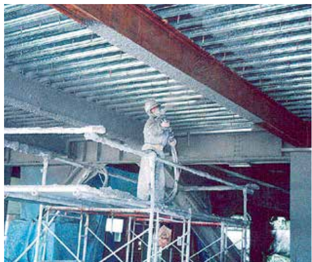
TOP: Reputable hardware (continuous mixer) is deployed; BOTTOM: A proper and safe job site setup is crucial in achieving the product’s designed in-place performance and in meeting the construction schedule.
